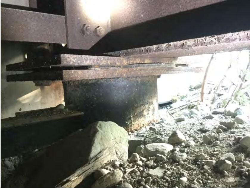
Typical Left Abutment Bearing - Bulging
